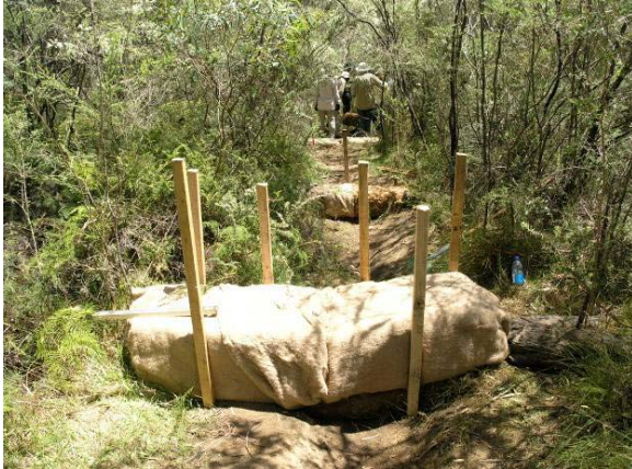
Plate 6-2 - Small Coir Log Dams Constructed at Intervals along an Incised Swamp with Jute Wrapping
